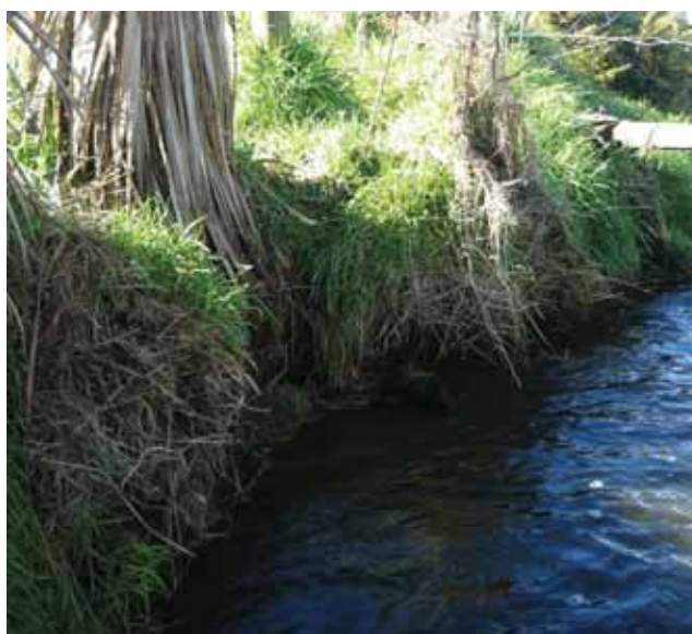
Bank has been undercut and the cabbage tree is vulnerable to falling in.
